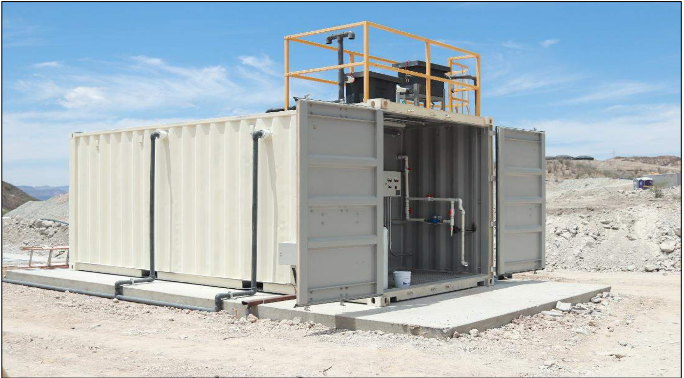
Figure 18-16: Sewage Treatment Module
