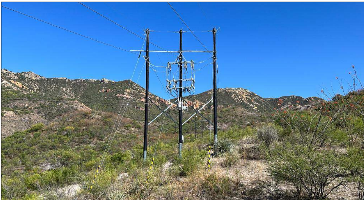
Figure 18-10: Electrical Power Line
