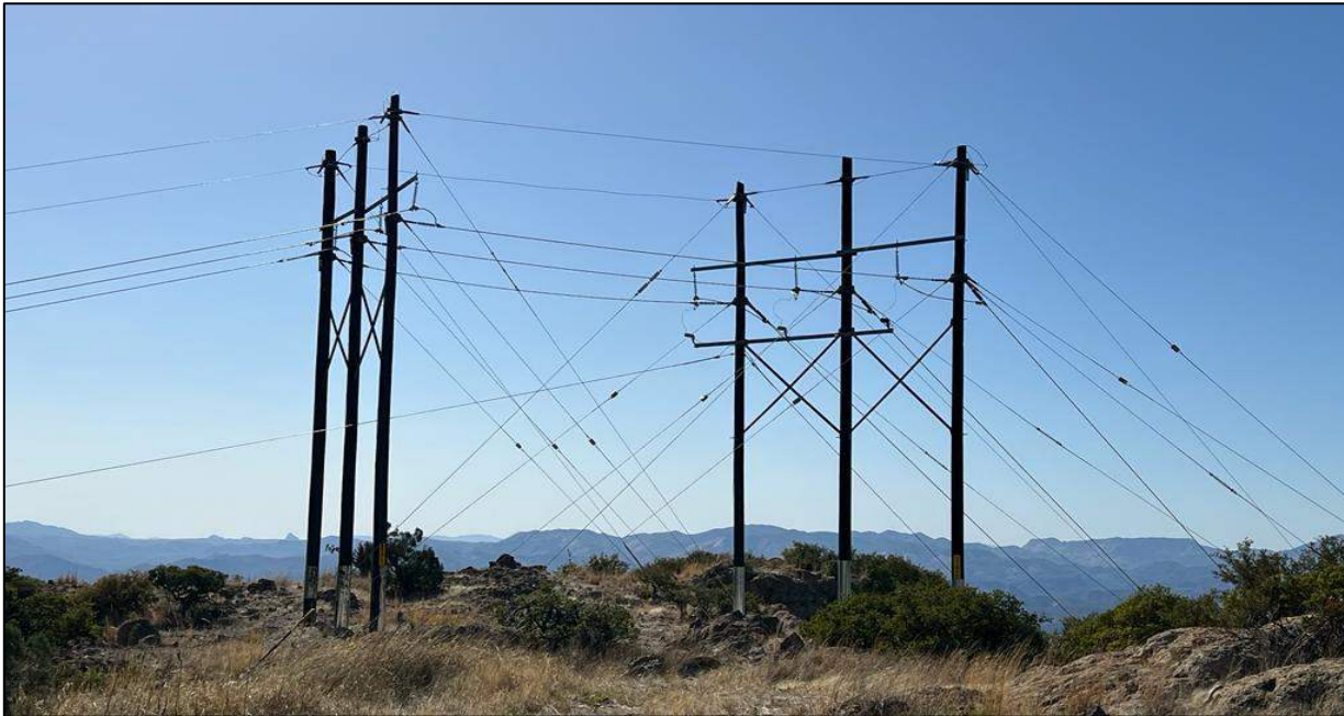
Figure 18-9: Electrical Power Line
