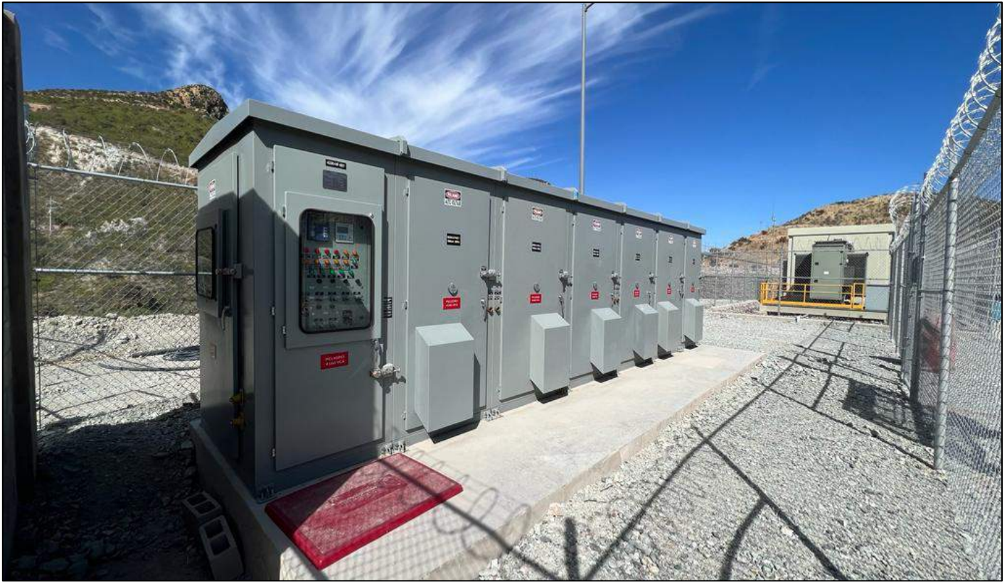
Figure 18-12: Power Equipment for 4.16 kV Distribution Bus
