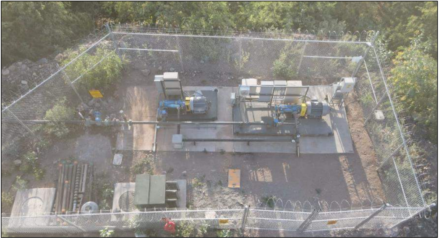
Figure 5-3: Sonora River Pumping Station
