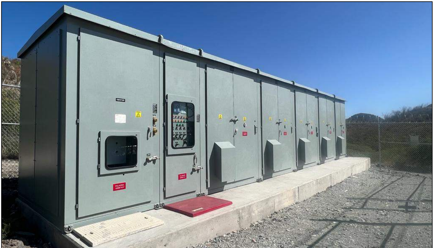
Figure 18-11: Power Equipment for 33 kV Line
